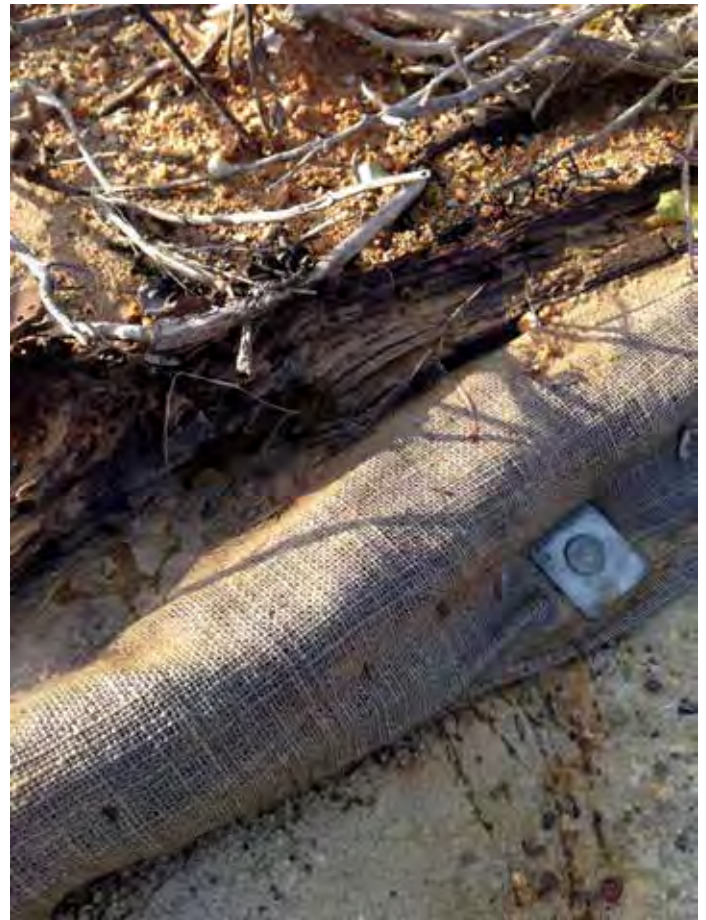
Photo 2: Hessian retained by roofing nails that have been driven into the soft bedrock
